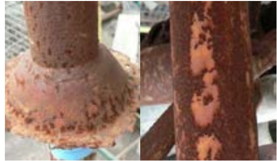
6. Deep rust, corrosion and pitting.
