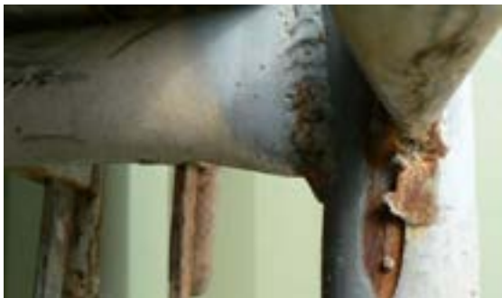
3. Cracked or corroded welds.
